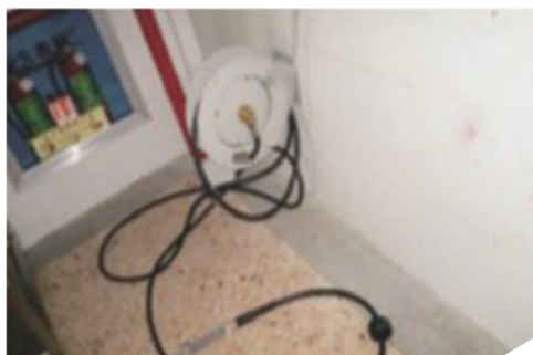
The installation height is too low and there is no recovery after reverse installation.
