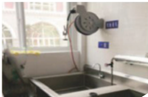
Installation height is not enough 1.3-1.6 m, the impact of easy to use collision.
